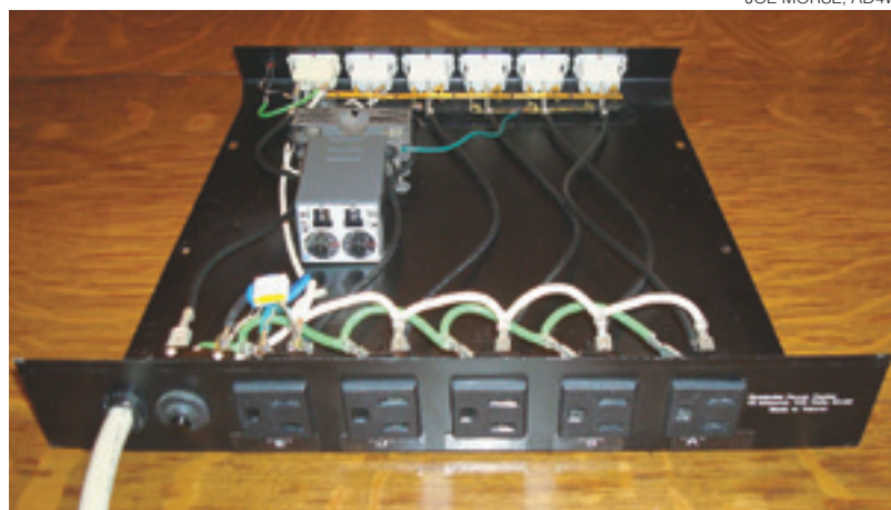
Figure 6 — Here is the computer power center with the timer installed.
